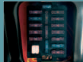
A concentrated fuse box for easy inspection
